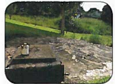
Keep septic tanks sealed.
